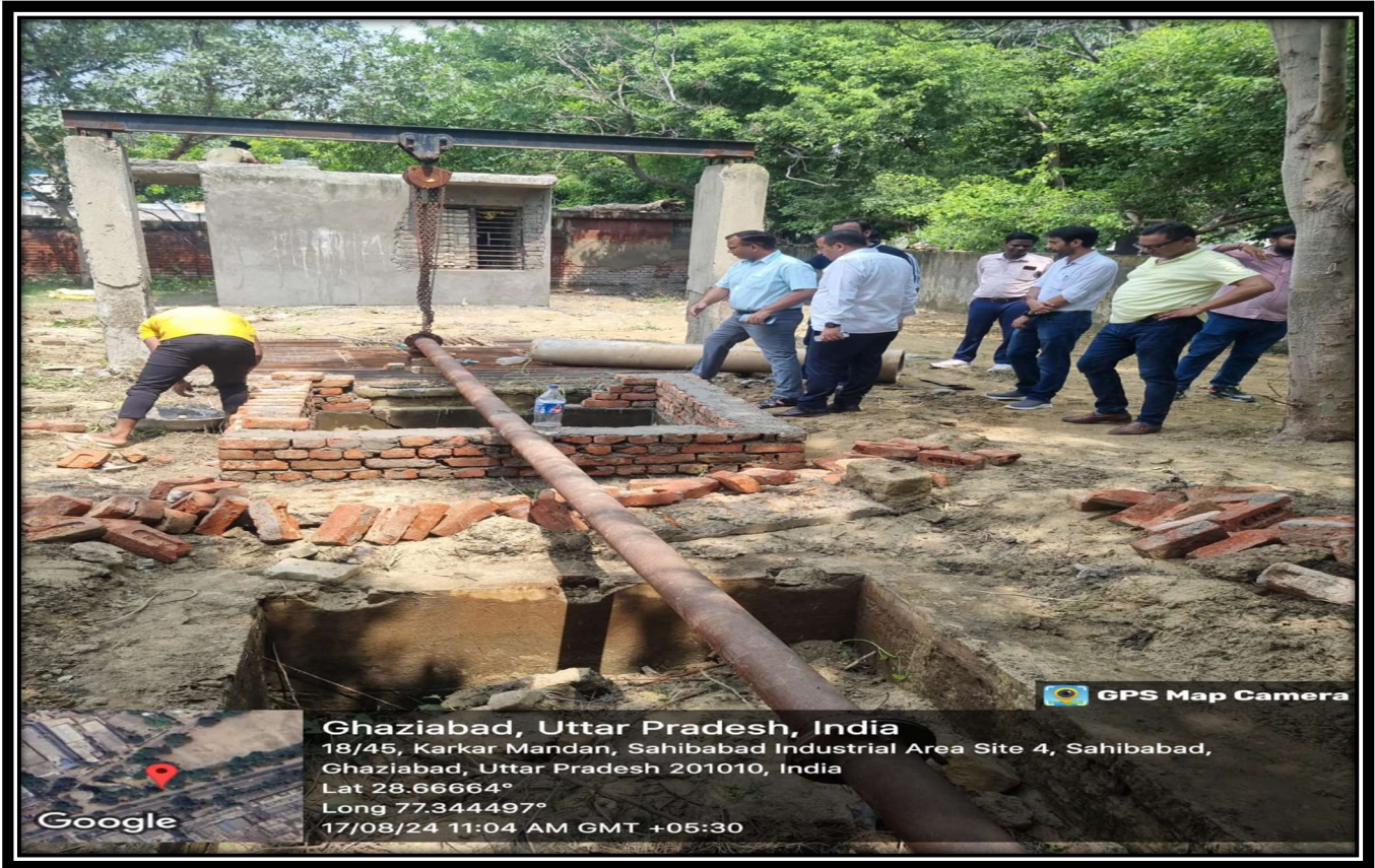
Existing pumping station with a temporary arrangement for pumping.
