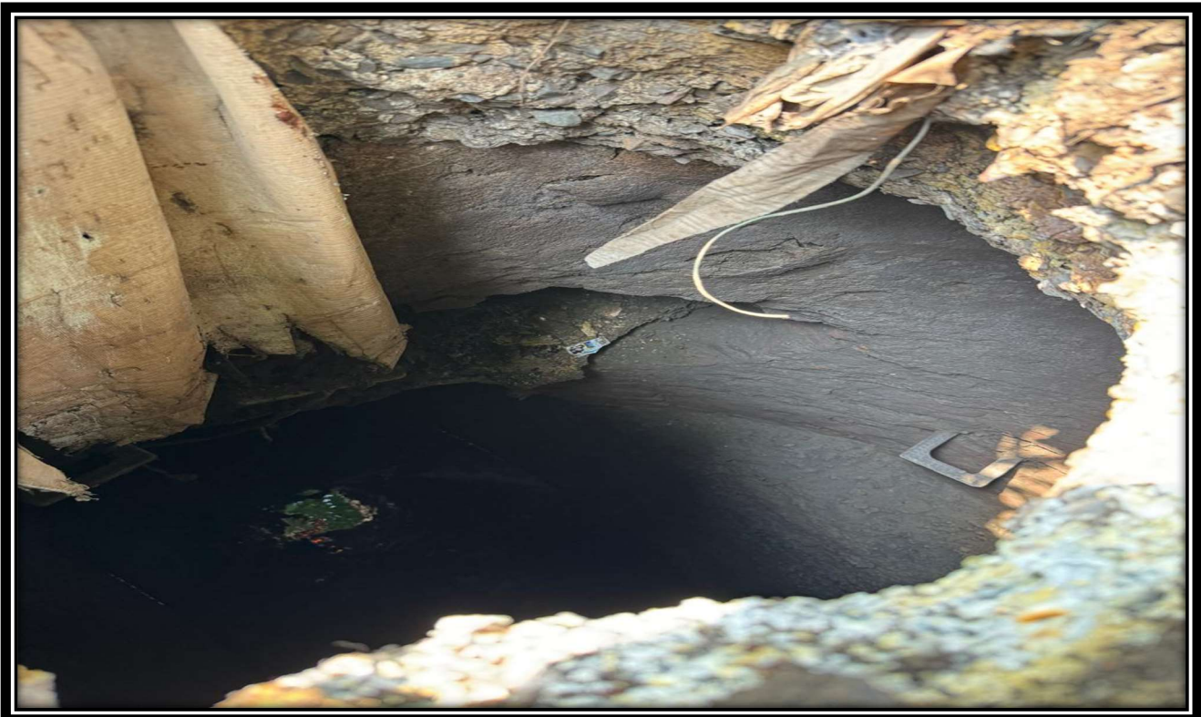
Common Chamber where rising main connected to trunk sewer line 1800 mm dia of 56 MLD STP Indirapuram
