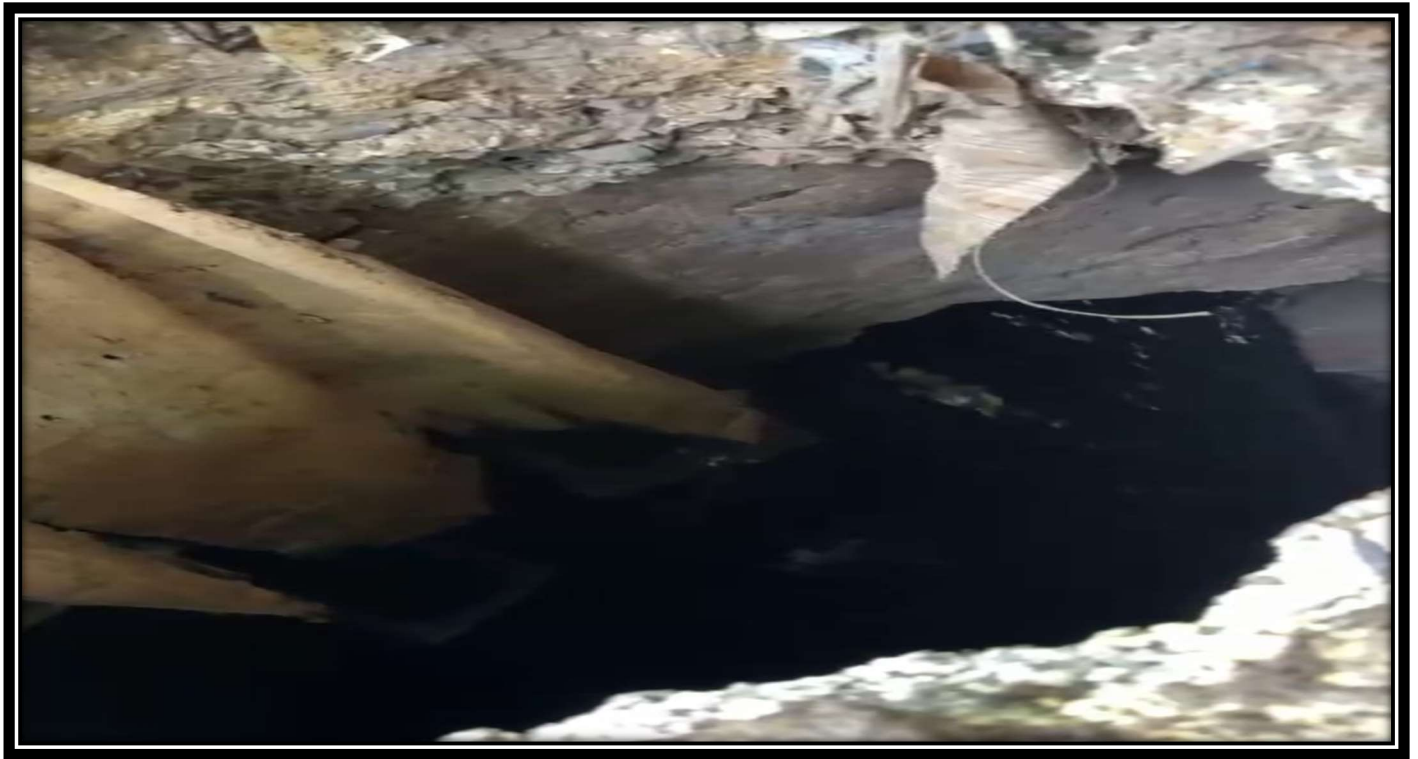
Free fall of sewage at common chamber from rising main into 1800 mm dia trunk sewer line of 56 MLD Indirapuram
